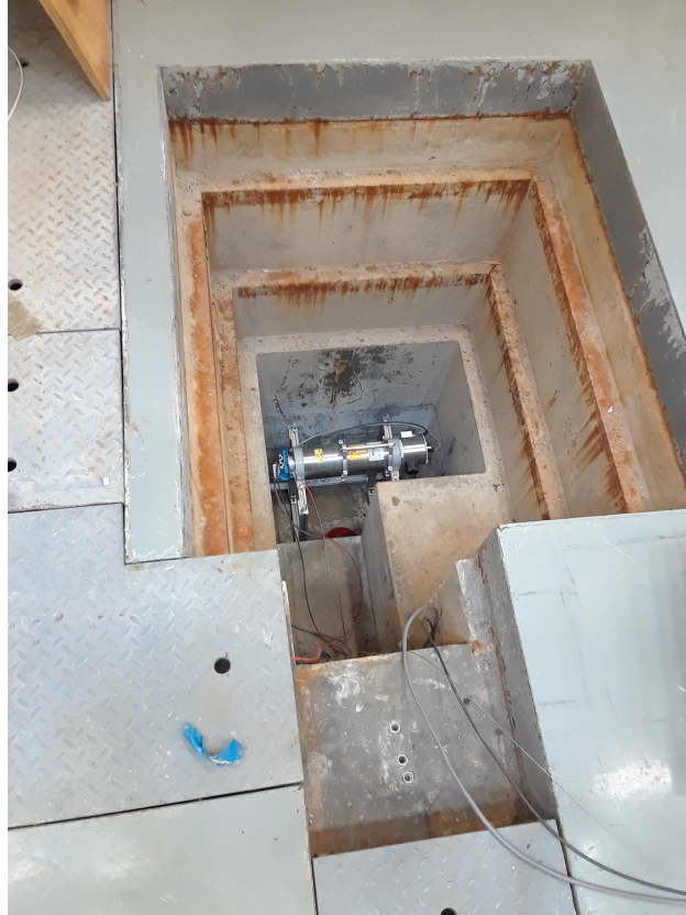
Figure 3.18: DT generator position in a pit, before it is covered with shielding
