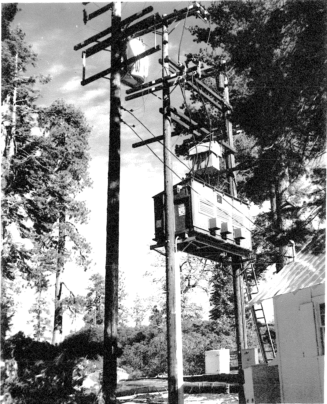
FIGURE G-4. TRANSMITTER BUNGALOW AND ASSOCIATED COUPLING EQUIPMENT.
